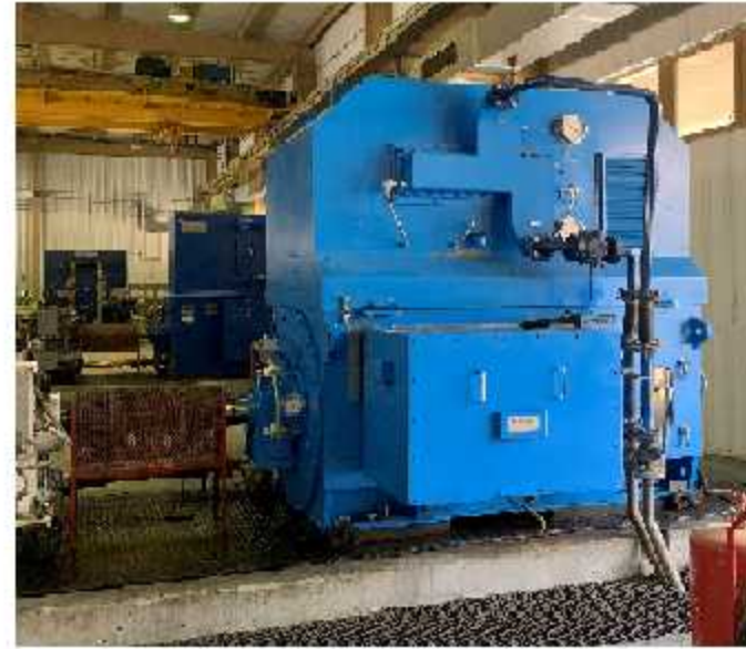
6150 kW Motor, 13.8 kV, 4 Pole Installed at a Desalination Plant Saudi Arabia
