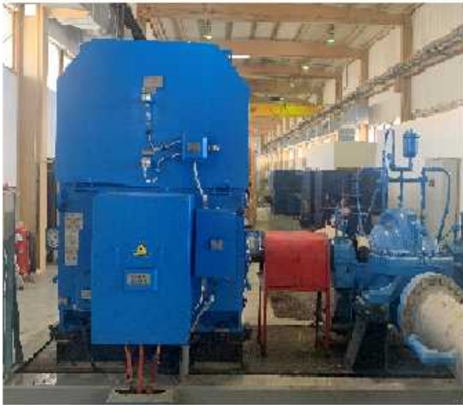
710 kW Motor, 4.16 kV, 2 Pole Installed at a Desalination Plant Saudi Arabia
