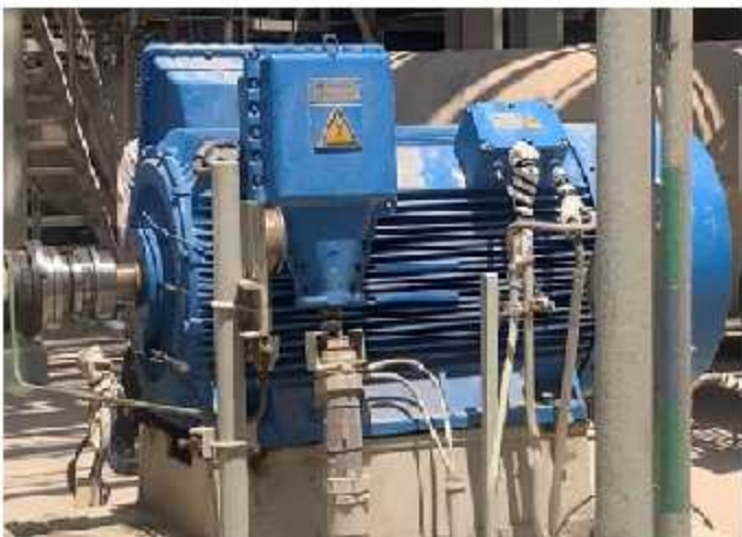
230 kW Motor, 4.16 kV, 2 Pole Installed at a Desalination Plant Saudi Arabia
