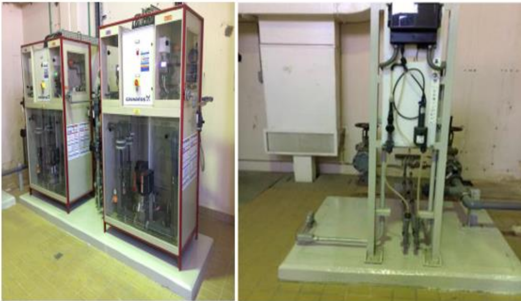
GRUNDFOS. Chlorine dioxide (ClO 2 ) Dosing Equipment Installed at SWCC Yanbu-Medina Pipe line
