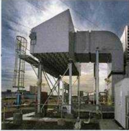
Air Intake System for Gas Turbine
